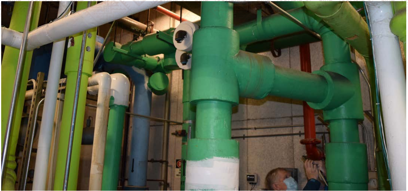
Beneath Boise's City Hall lies an intricate network of pipes that act as a heat exchanger for the city's geothermal district heating systems. Idaho workshop participants toured the mechanical room at City Hall to view the infrastructure.
