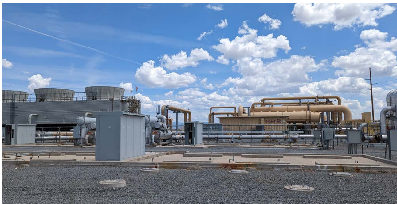
Cymru Energy's Thermo Geothermal Power Plant, which sustainably produces power used in Anaheim, California.
