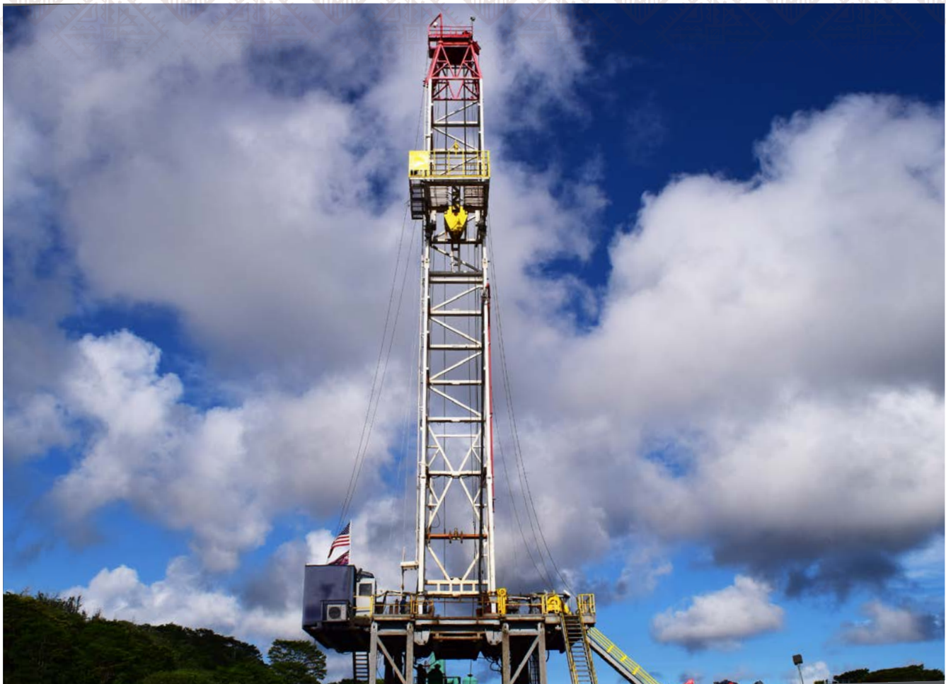
Preparing for drilling at the Puna Geothermal Venture, operated by Ormat Technologies Inc. The exploration and drilling phases often bring the highest risk for failure and the most cost to geothermal development.
