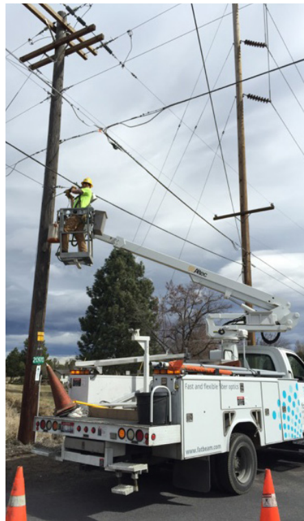
Idaho-based Fatbeam installs fiber-based networks, such as this one, that help expand broadband connectivity in the West.
